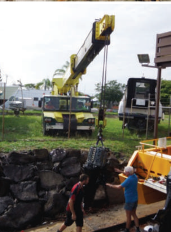
FROM TOP: Excavator coming down. Re-positioning rock for ramp repair. Off with its head!
