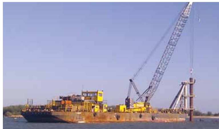
Contractor's barge replacing navigation marks in the Burnett River. Note the rock wall is not papier mache!
