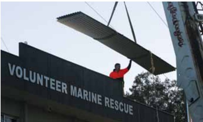
Roofing materials were lifted by crane onto the base roof. Photo by Peter McNamara
