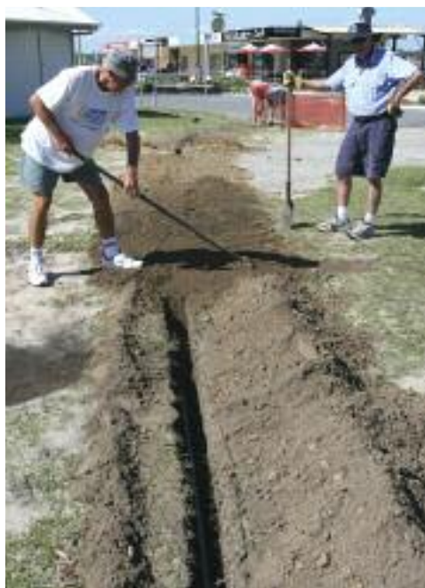
left: You always need a few good men on shovels when your digging a trench to lay the cable for the CTV cameras from the pontoon to the base. Tex Howarth and Neil Plumb show their style at the working bee hold on Wednesday November 21, 2012.
