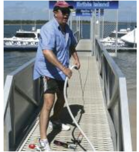
right: New Radio Operator Andy Joyce helping at the working bee on Wednesday November 21, 2012 when a trench had to be dug to lay the cable for the CTB cameras from the pontoon to the base. Andy seen here working on connecting the new cable along the pontoon to the cameras
