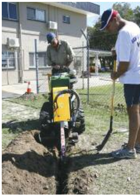
left: Clint Fullgrabe driving the trench digger at the working bee on Wednesday November 21, 2012 when a trench had to be dug to lay the cable for the DTV cameras from the pontoon to the base.
